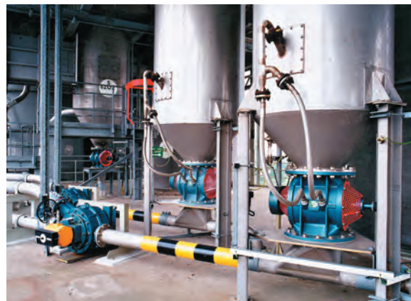
Product feed from silo via rotary valve.
